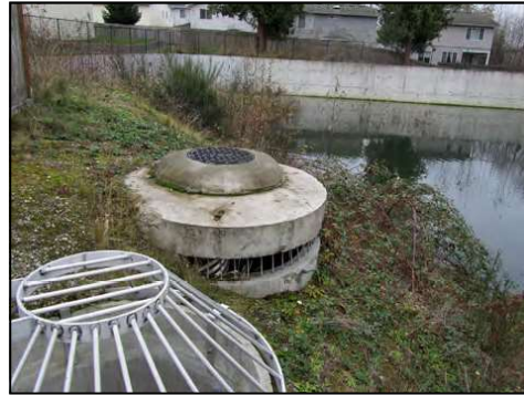
Typical detention facility with control structures.
