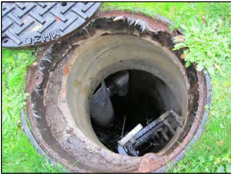
Typical manhole access to control structure.
